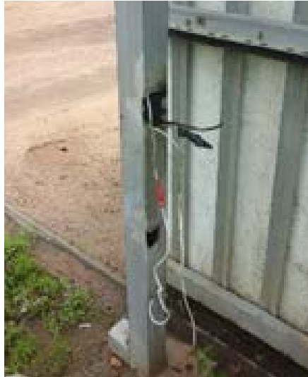
Gate motor stolen at Groot Drakenstein cultural facility in Simondium.
